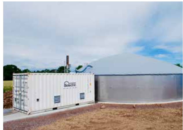
Bioelectric | Biogas installation
