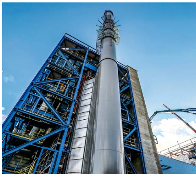
The new gas and steam turbine power plant under construction in Marl (Germany).
