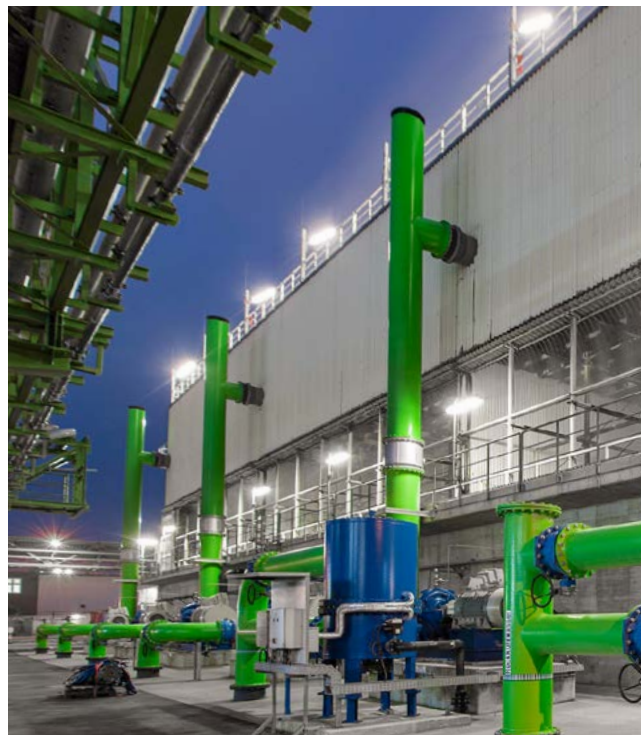
Wesseling (Germany): A cooling tower made of glass-fiber-reinforced plastic reduces the temperature of cooling water after use. Some of the water can be re-used in the cooling system.
