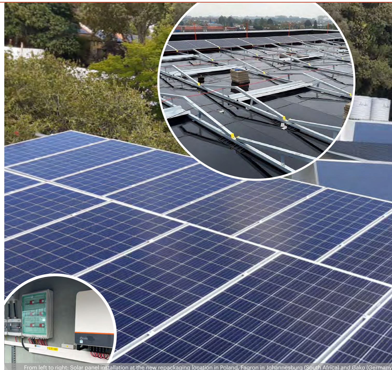
From left to right: Solar panel installation at the new repackaging location in Poland, Fagron in Johannesburg (South Africa) and Gako (Germany).
