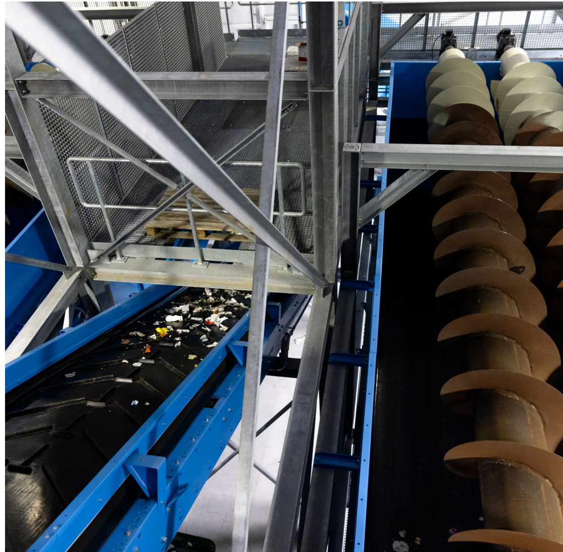
In the new pretreatment installation in Willebroek, we prepare sorted PMD waste for recycling into new raw materials.
