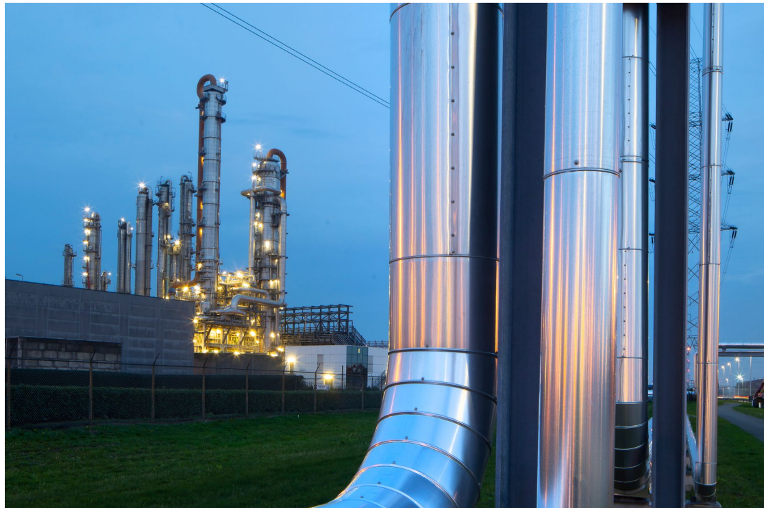
Steam network ECLUSE supplies green energy from the Waste-to-Energy installations in Doel (BE) to industrial parties.
