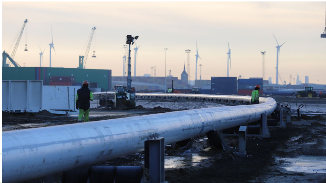
A pipeline gets the residual heat from our rotary kilns to Boortmalt.
