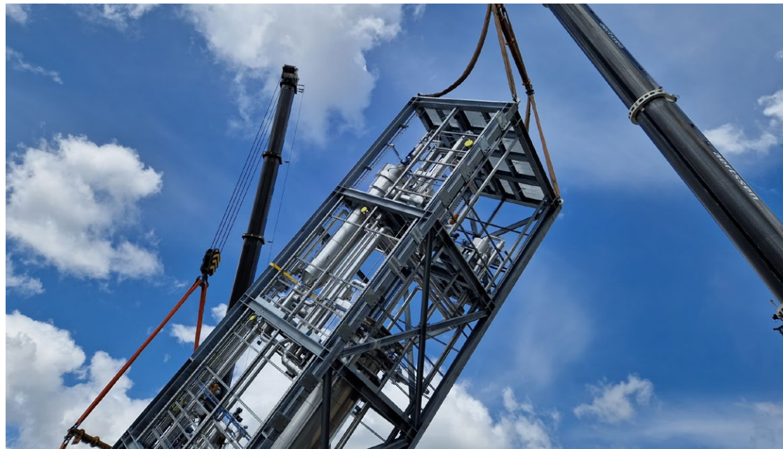
Construction of the innovative demo plant for the chemical recycling of complex plastics.
