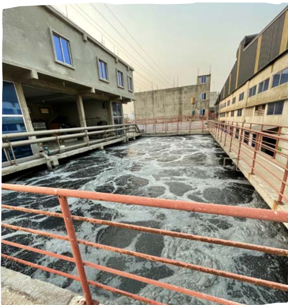
Photo of a water treatment system at one of our suppliers participating in the Better Mill project.
